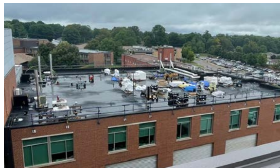
Here is a picture of the Tower B roof work. Tuesday was a rain day, but the contractor will be back as soon as weather permits.
