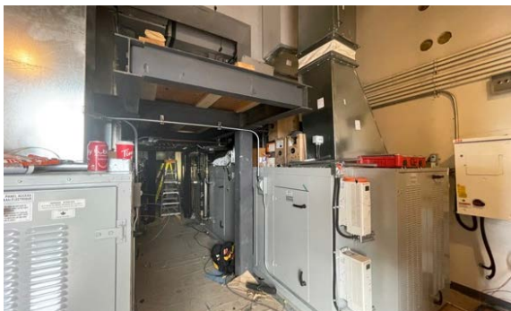
This is the mechanical room which is still a very busy area. We are very close to seeing the testing of the new air handling units.
