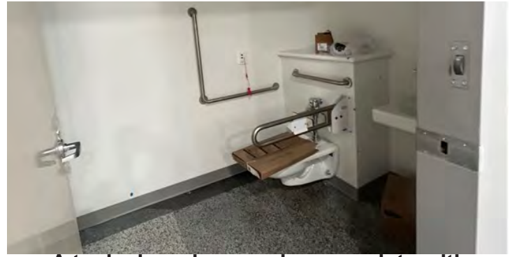
A typical washroom also complete with a UV system.
