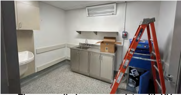
The new soiled room complete with UV sterilization light.
